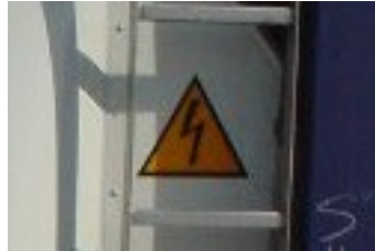
Figure 8.5 Overhead warning sign
