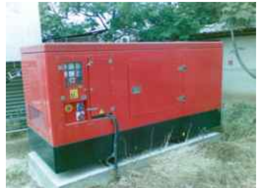
Maintain generators in good condition
