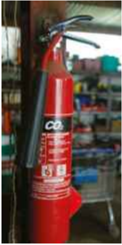
Fire extinguishers should be close to hand
