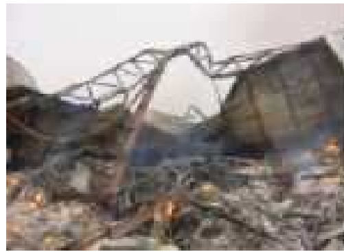
Collapse of the lattice beams of the large storage cell
