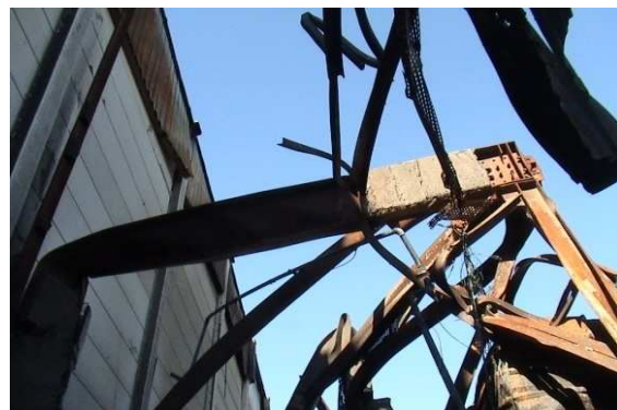
d) Structure components after the fire
