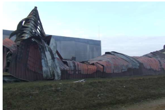
b) Collapse of the structure inside the cell
