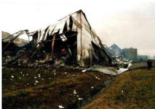
Collapse of the large storage cell towards the inside of the building
