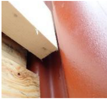
Figure 10-76 Beam too short
