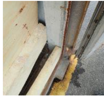
Figure 10-77 Beams too short
