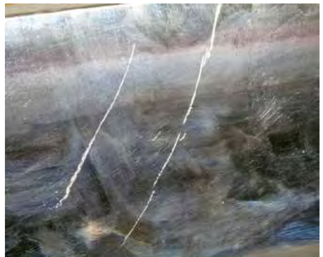
Figure 2. Scratches on a stainless steel tank surface.
