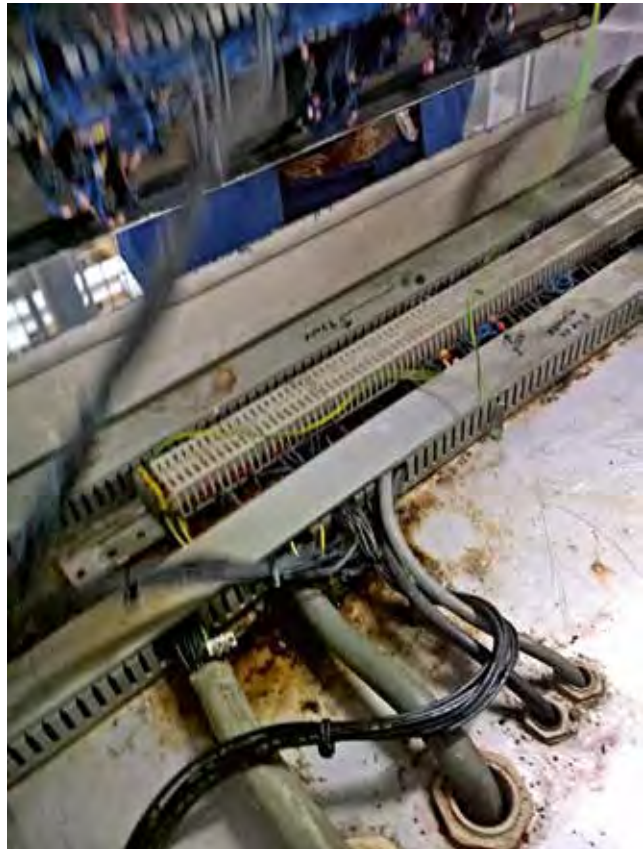
Figure 4. Bacteria spreading in non-pressurised equipment.
