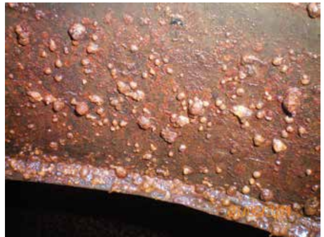
Figure 7. Electrolytic corrosion due to electrical exchanges between two different types of metal, enhanced by the presence of detergent solutions.
