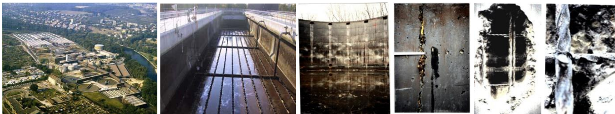
Figure 7.4 Assessment and rehabilitation of large scale prestressed concrete basins and tanks in an urban sewage-treatment plant
