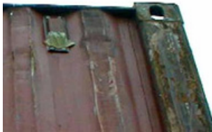
Figure 5.20 Vent tapped over
