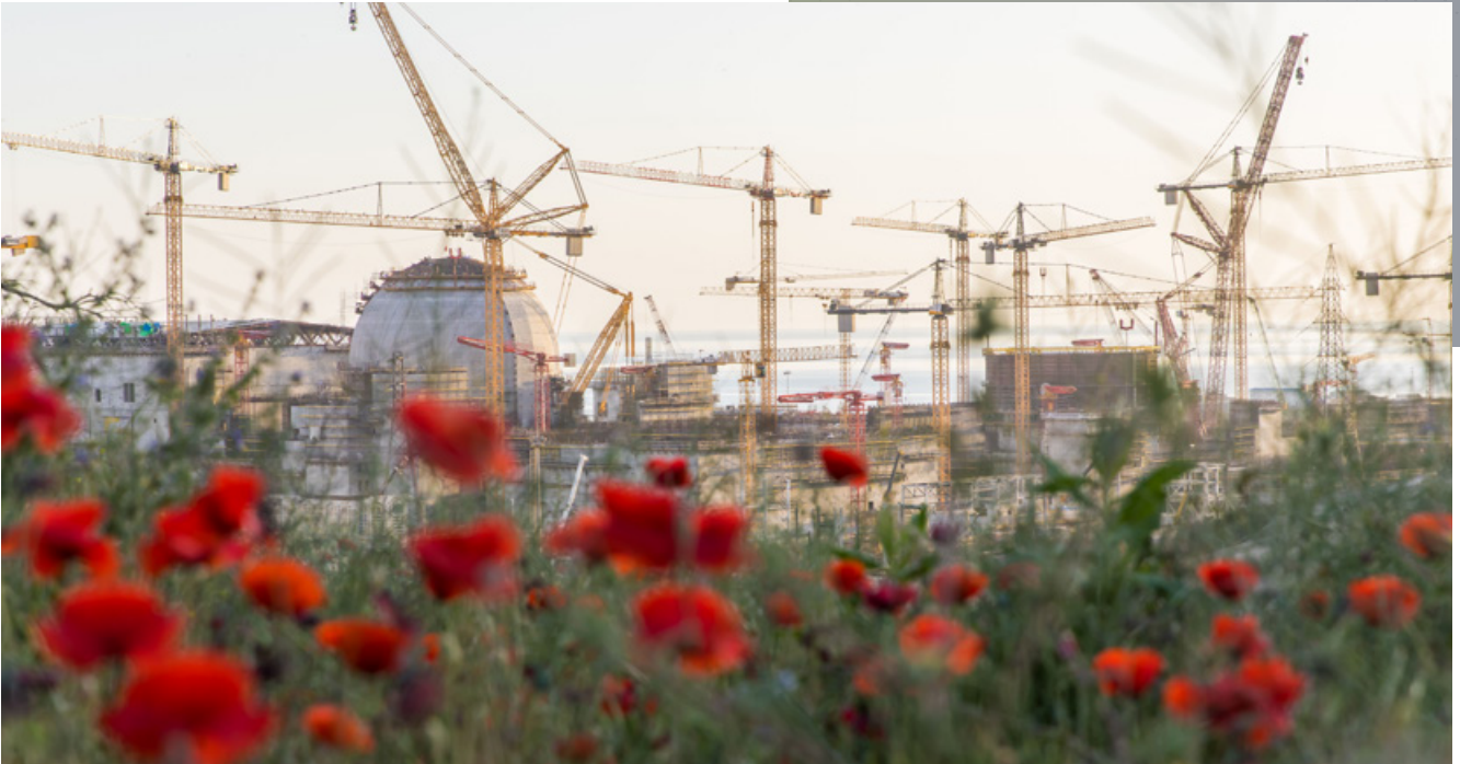
Akkuyu nuclear power plant, Türkiye. Courtesy of Akkuyu Nuclear Joint Stock Company
