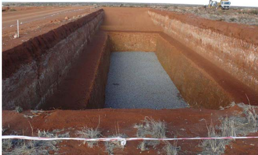
FIG. 3. Near surface trench at Vaalputs. Courtesy of National Radioactive Waste Disposal Institute.
