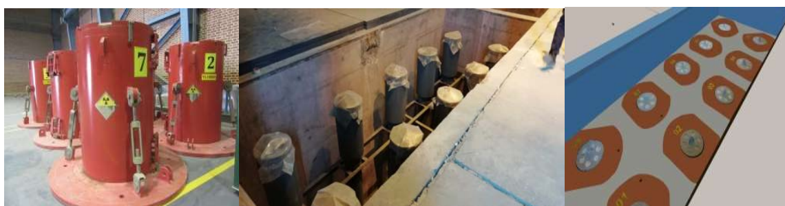
FIG. 3. New boreholes for long term storage of steel capsules (highly active solid waste).
