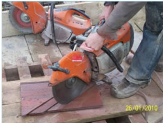
Good practice – Cutting roofing tiles with a tile cutter (National Federation of Roofing Contractors Ltd, GB)
