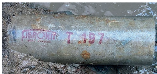
Image 1 Cutted asbestos-cement water pipe still in place
