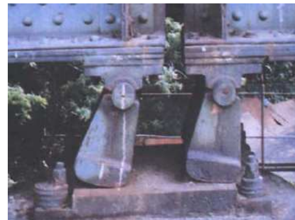
Fonte: BRIDGE INSPECTION MANUAL – NY'S DOT
