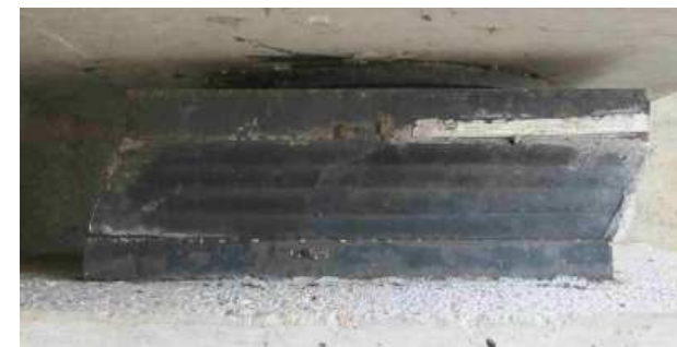
Fonte: BRIDGE INSPECTION MANUAL – NY'S DOT
