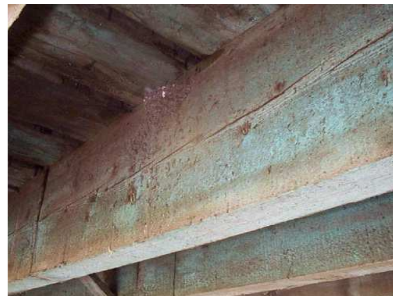
Fonte: BRIDGE INSPECTION MANUAL – NY'S DOT
