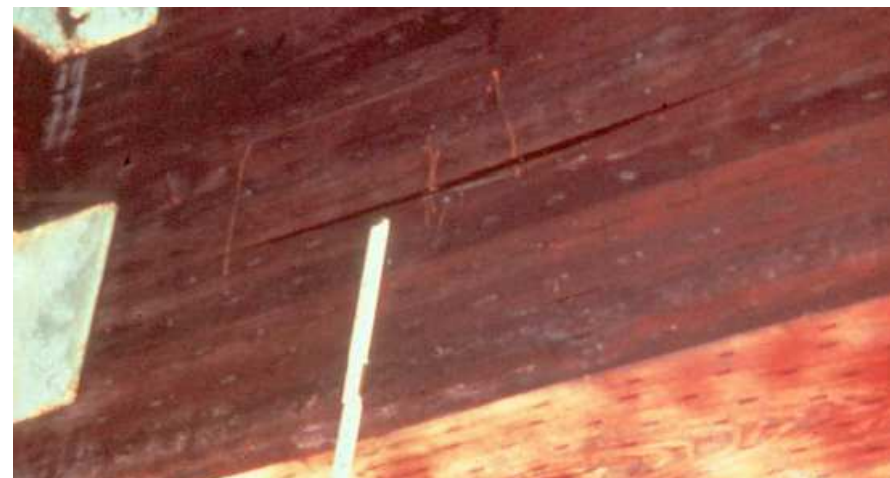
Fonte: BRIDGE INSPECTION MANUAL – NY'S DOT
