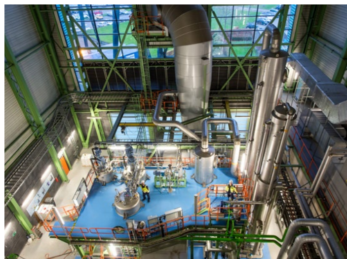
A pilot CO 2 capture and utilisation plant at Twence Waste-to-Energy plant. Image courtesy of Twence.
