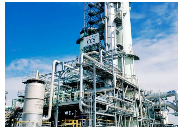
Top: Tomakomai Demonstration Facility. Image courtesy of Japan CCS Co., Ltd. Above: Mikawa Power Plant. Image courtesy of Toshiba Energy Systems & Solutions Corporation (Toshiba ESS).
