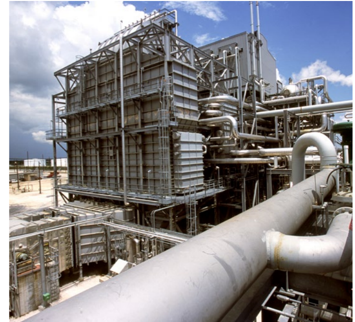
Air Products' Port Arthur Texas Hydrogen Plant. Image courtesy of Air Products and Chemicals, Inc.
