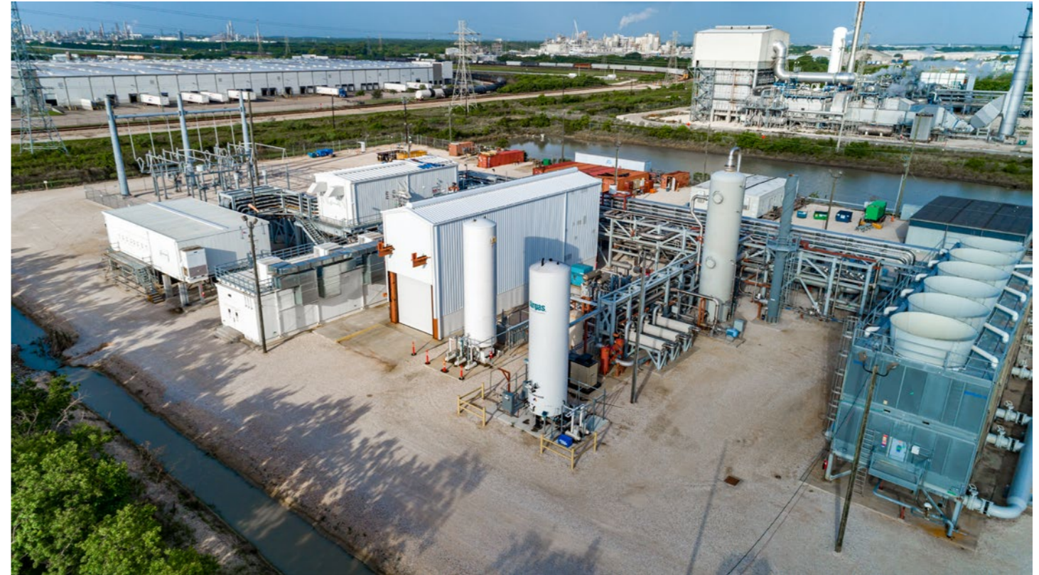
NET Power's Pilot Project in La Porte, Texas. Image courtesy of NET Power.
