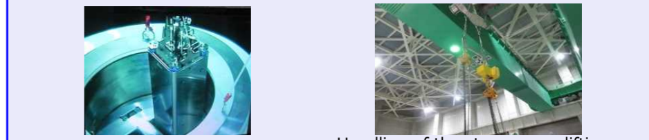
<Lifting of the storage can> <Handling of the storage can lifting tool at the main hoisting>
