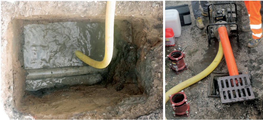
Figure 4 - Channelling the water at the bottom of the dig and discharging into the sewer.
