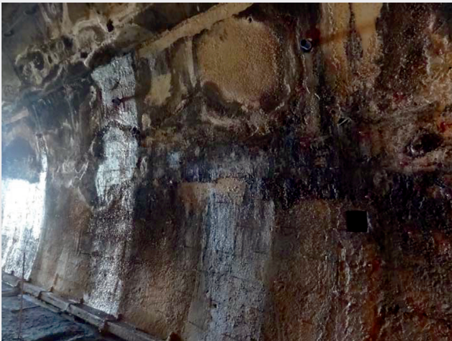
Fig. 10. Fessure diffuse, bagnate
