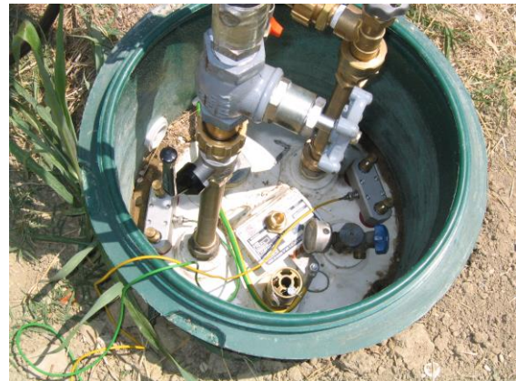
Figure 11. A view of the locker of a small underground tank for AE test
