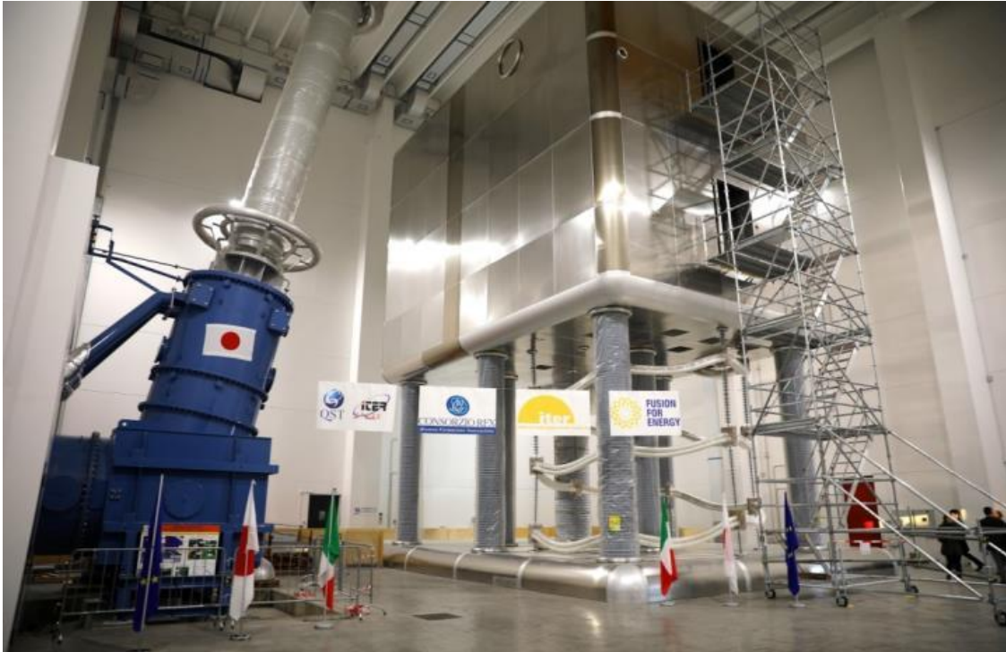
Figure 5. MITICA High Voltage Hall
