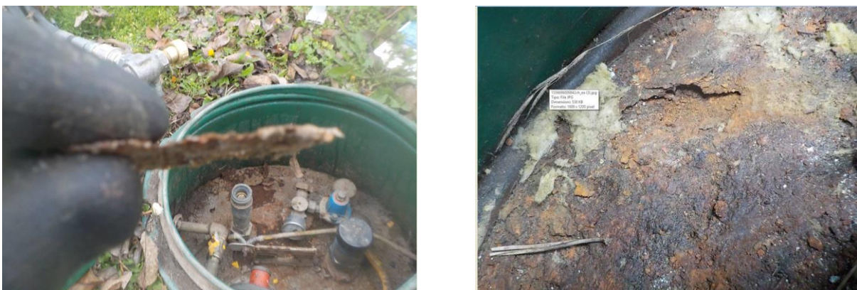
Figure 32. Evident advanced corrosion on a GPOL vessel. AE test shall not be performed
