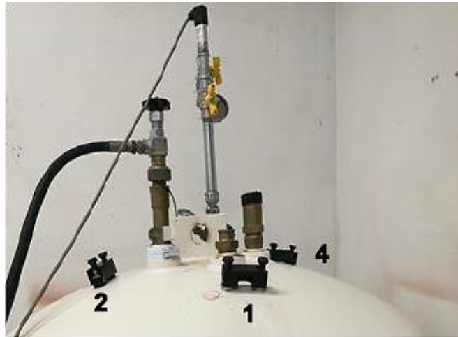
Figure 2 – Sensor placement on the top of the tank
