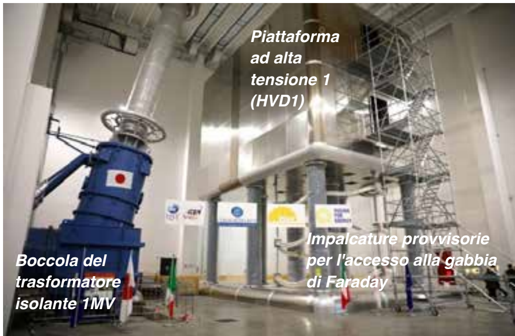
Figura 6. MITICA High Voltage Hall
